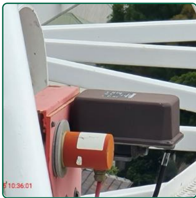
Trolley In and Out Limit Switches
