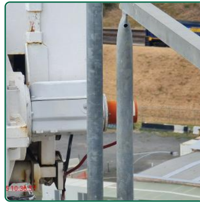
Hoist Upper and Lower Limit Switches
